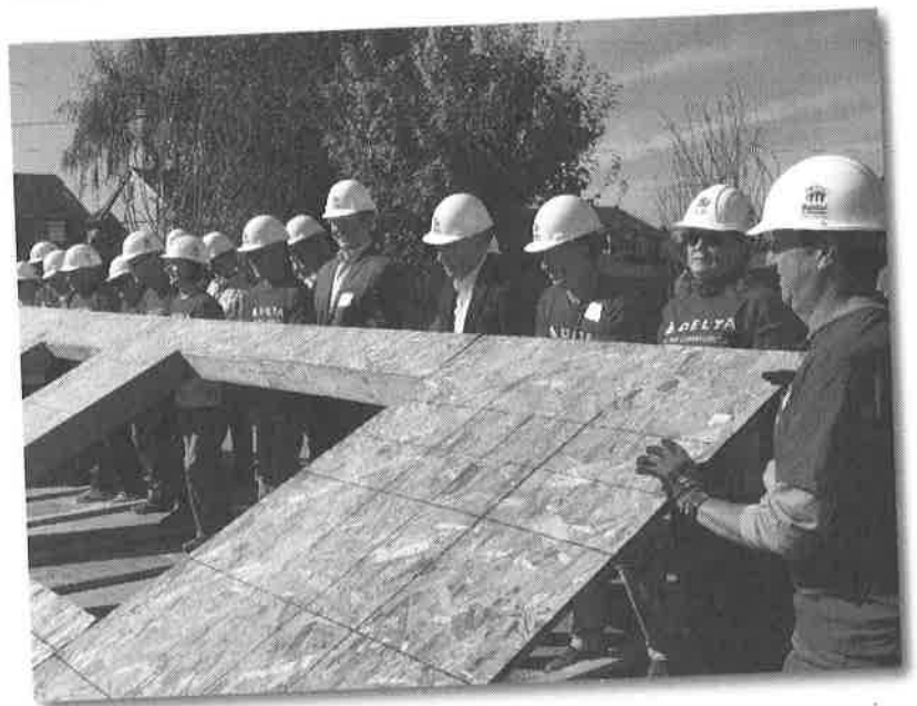
Raising the wall for one of nine Habitat for Humanity Blitz Build homes for veterans in Pacific.
